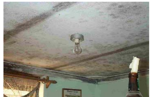
Mould growth on a ceiling
